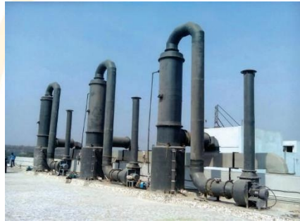
PP-FRP Scrubbing System
