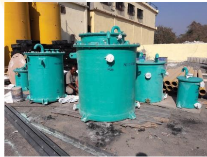
FRVS Dosing System Tank
